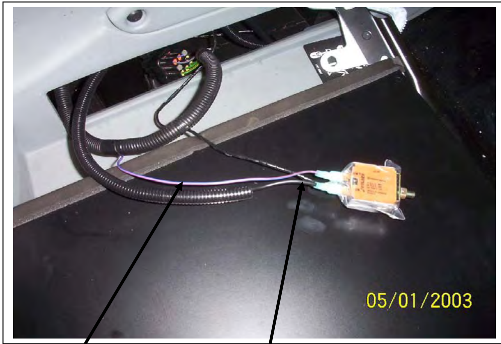
Wire from A/C switch on control panel.
