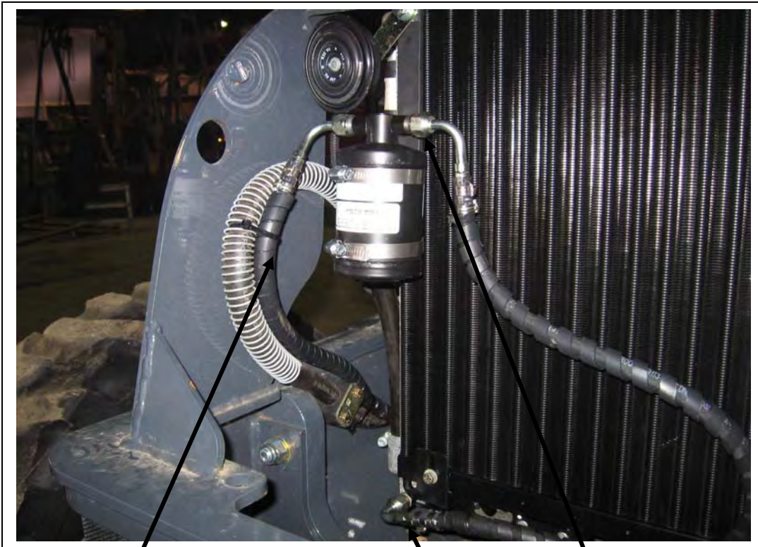
5/16" 90° fitting at drier outlet on long 5.16" hose.
